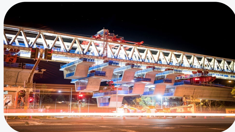
SEGMENTAL PRECAST BOXED GIRDERS
