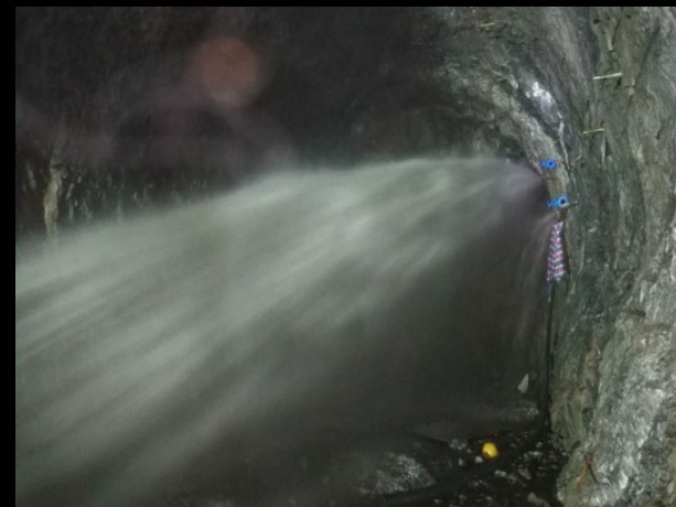
T6+763m Serious water gushing on the face of the tunnel
