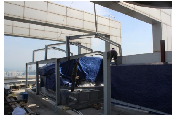
Control Room Frame
